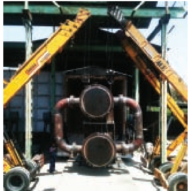
PWHT Heat Exchanger
